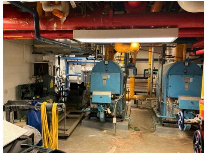
28 - MAIN MECHANICAL ROOM
