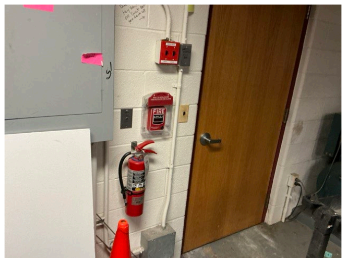
36 - FIRE EXTINGUISHER AND ALARM DEVICE
