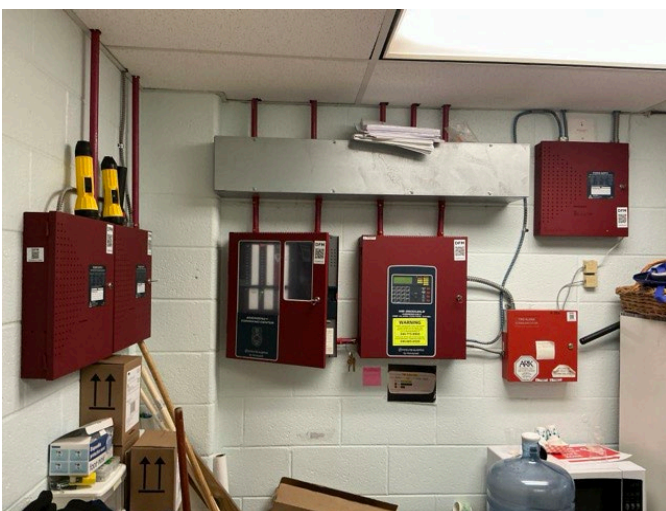
35 - FIRE ALARM PANEL
